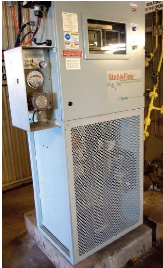
Figure 3. A pair of Nel Hydrogen StableFlow gas control systems to maintain optimal gas dryness, pressure and purity inside the generators.
