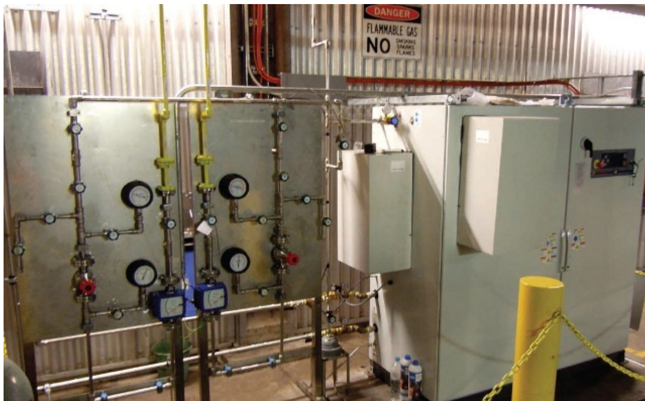
Figure 2. NPS installed a Nel Hydrogen H-Series hydrogen generator, which produces 2\text{Nm}^3 of ultra pure cooling gas each hour, using only electricity and deionized water.
