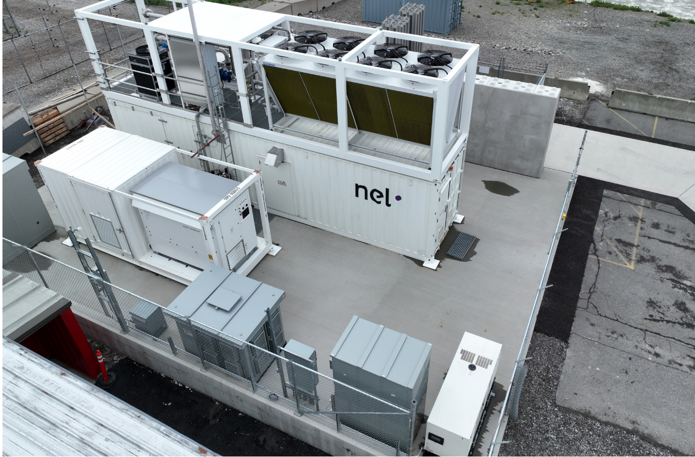
A Nel Hydrogen containerized PEM Electrolyser IMAGE: CONSTELLATION ENERGY CORPORATION
