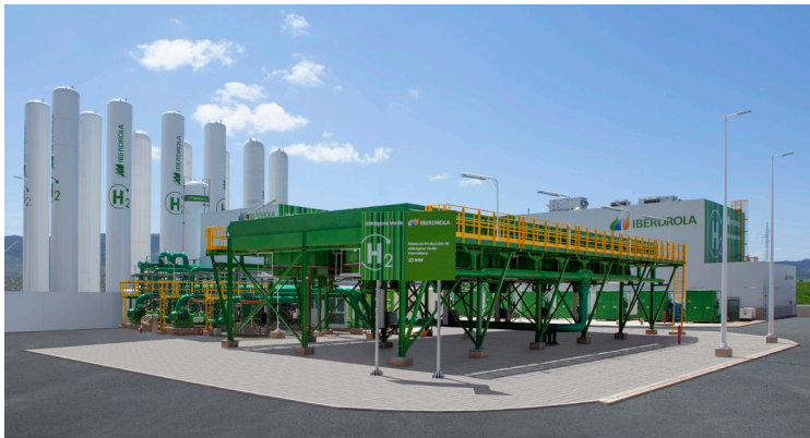
Figure 2. The 20 MW PEM plant at the Iberdrola-Fertiberia facility in Puertollano, Spain, featuring Nel electrolysers, is the largest electrolysis plant currently in operation providing green hydrogen for green ammonia production.
